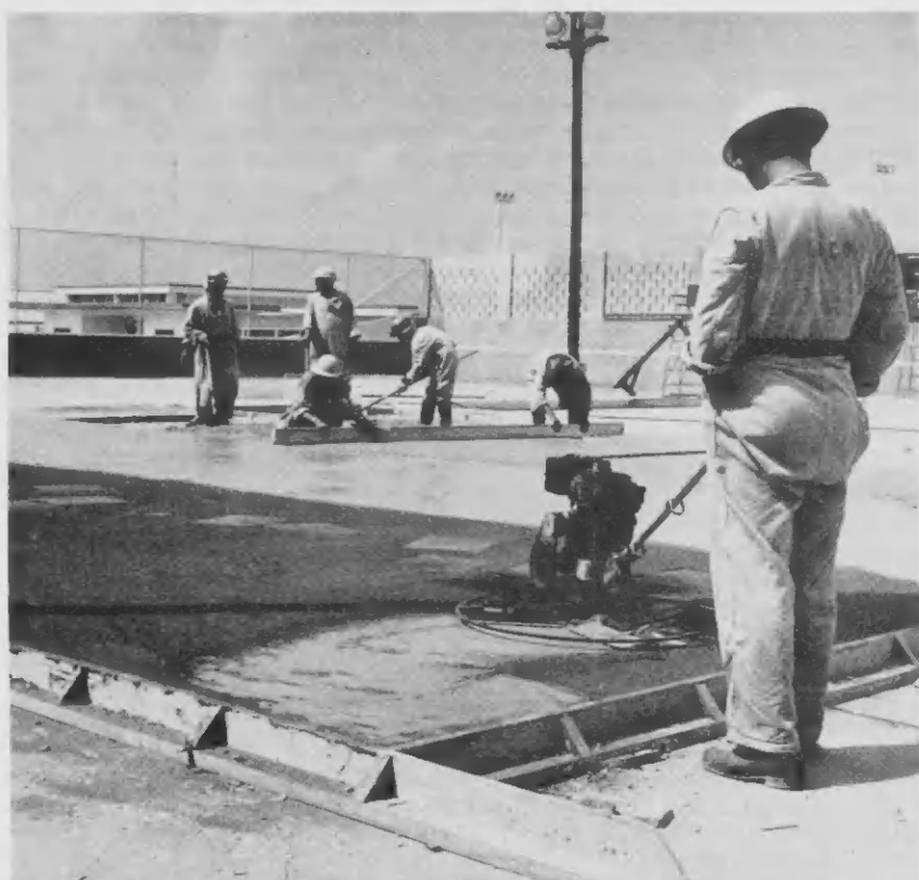
COLOR IS added to the concrete after it has been poured. It is spread by a mechanical float mixer which works the concrete in a manner that allows the color to permeate the mixture. The court slab at the Lago Sport Park is green.
